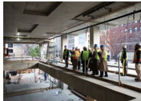
Members of the GW community toured the Science and Engineering Hall in December to celebrate the completion of the initial concrete structure.
