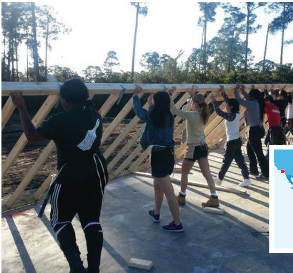
GW volunteers in Indian River County, Fla., lift the framework of a house into position during their service project with Habitat for Humanity.
